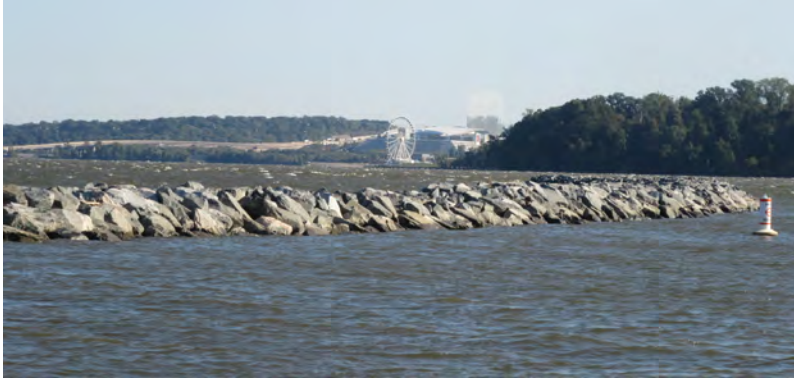
The completed breakwater with a view of National Harbor's ferris wheel on the Maryland side of the Potomac River.
