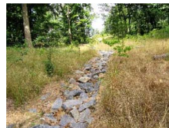
The completed restoration has riprap, plunge pools and native plants and trees. Photo by Glenda Booth
