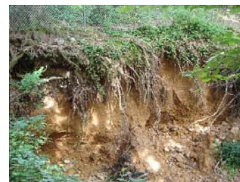
The failing outfall in Mount Vernon District Park, 2014, gouged out streambanks. Photo by Glenda Booth
